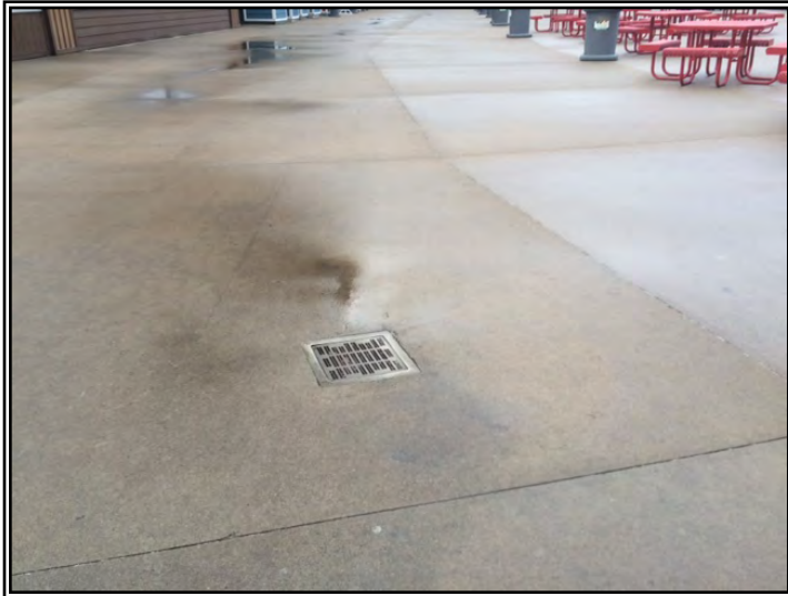
Area Drain on Concourse Level
