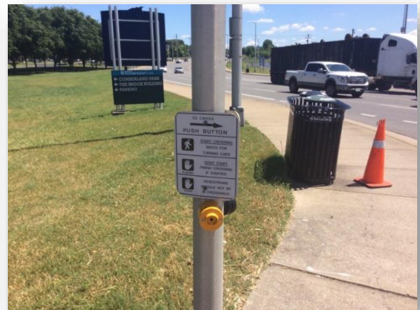
Push button cannot be initiated with fist, South 2 nd Street and Shelby Avenue
