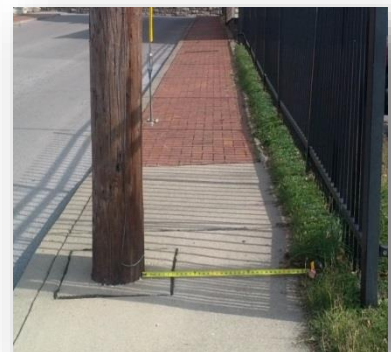
This pole is in the way of path of travel. You measure from the edge of the pole to the edge of the concrete.
