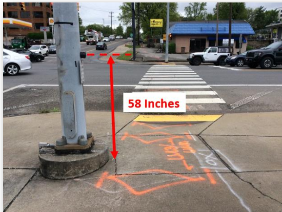
Push button that exceeds the height requirements, Harding Pike and White Bridge Pike
