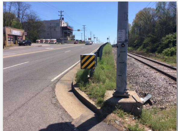
Pedestrian signal with failed landing requirements, Old Hickory Boulevard and Park Circle
