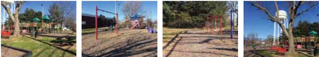
Equipment is older but in good condition. Surfacing requires routine maintenance to ensure proper depths. Layout and materials do not meet current ADA guidelines for accessibility.
