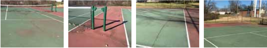
The existing courts have extensive cracking and are in need of resurfacing. They are also not regulation size.
