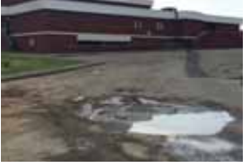
The existing parking does not have accessible routes to the building and pavement is in poor condition.
