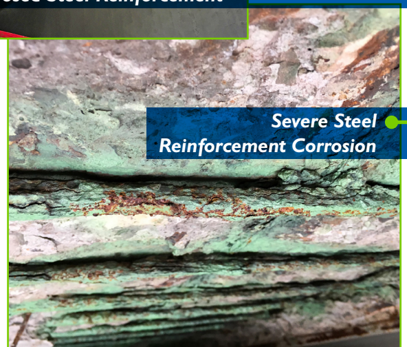
Delaminated Bridge Deck Concrete w/ Exposed Steel Reinforcement
