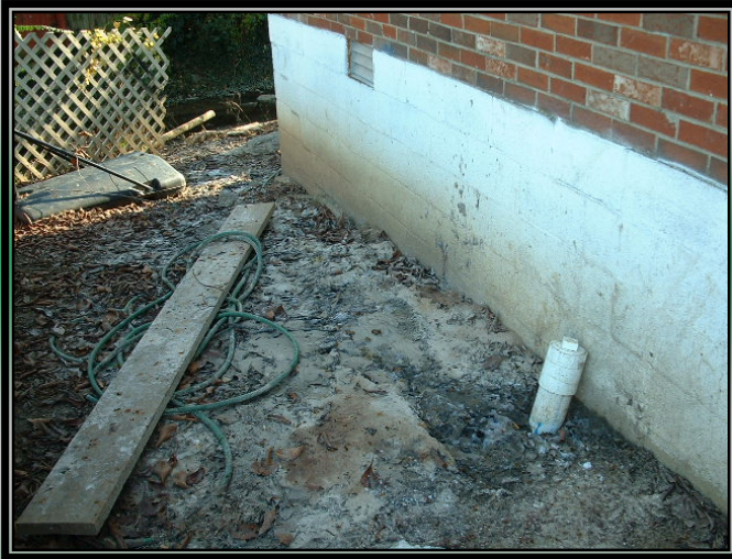
Broken or overflowing sanitary sewer cleanouts
