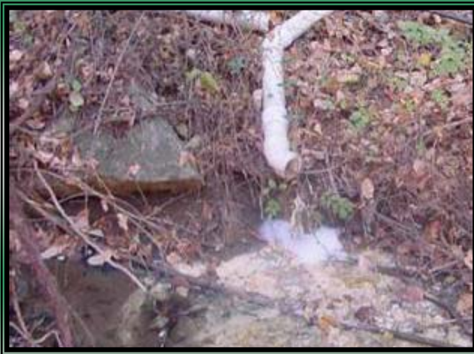
Illegally plumbed sanitary drains to creeks or storm drains
