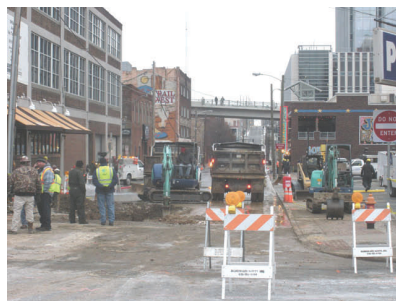
36" Main Break on 2nd Avenue South
