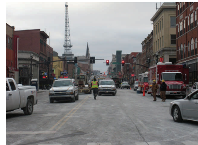
24" Main Break on Broadway between 4th and 5th Avenues
