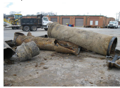
Damaged 36" water main pipe
