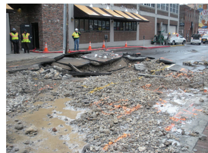
In front of Big River Grille & Brewing Works-road damage caused by the 36" water main break on 2nd Ave South
