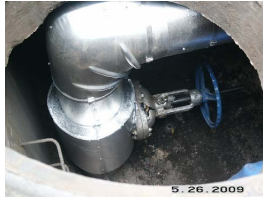
Manhole 6A New Steam Valve and Insulation
