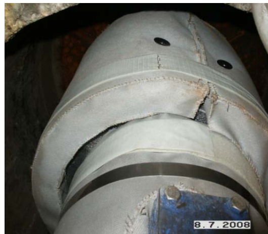
Temporary Boiler Insulation Blanket
