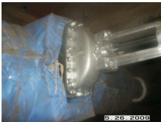
Manhole 13 New Steam Valve
