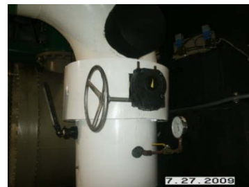
#6 Chiller Evaporator Outlet Valve
