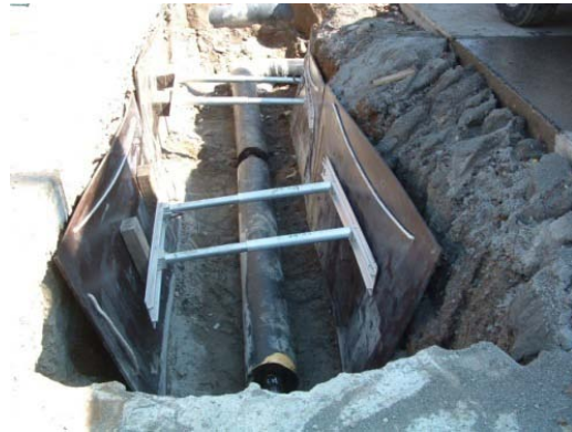
Manhole B to Symphony Condensate Line
