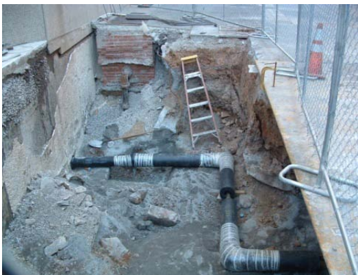
Citizen's Plaza Condensate Service Piping
