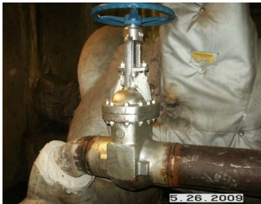
Manhole 23 New Steam Valve
