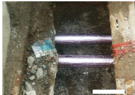
401 Union Condensate and vent lines
