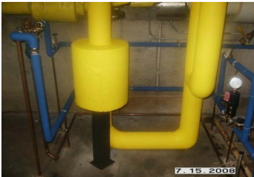
401 Union Condensate Flash Tank and Piping
