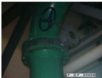
#4 Chiller Condenser Valve
