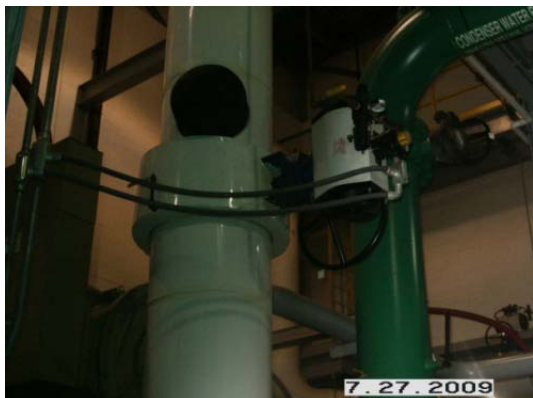
#3 Chiller Evaporator Inlet Valve
