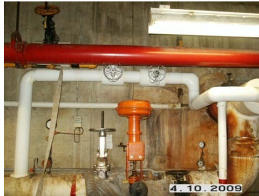
State Steam Tunnel PRV Bypass
