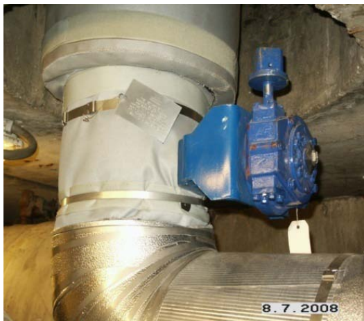
Temporary Boiler Isolation Valve
