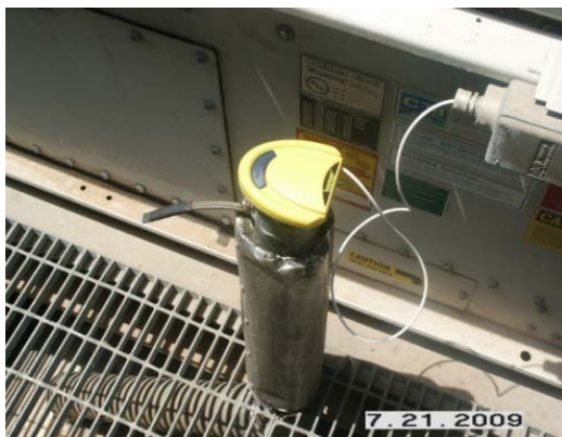
Old Sonic Level Transmitter
