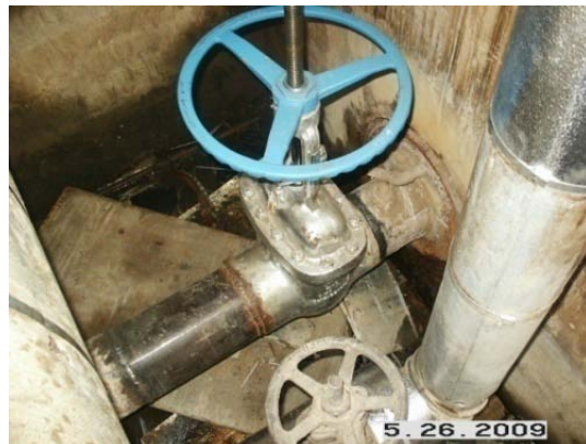
Manhole B New Steam Valve
