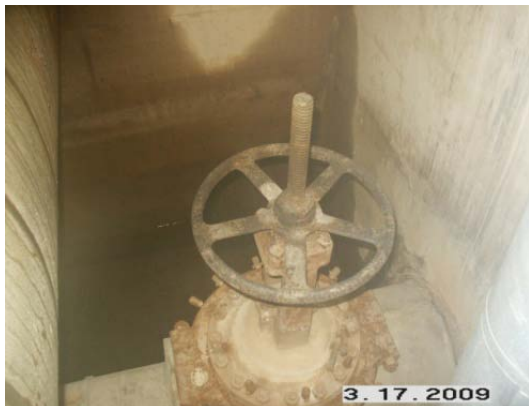
Manhole B Existing Steam Valve
