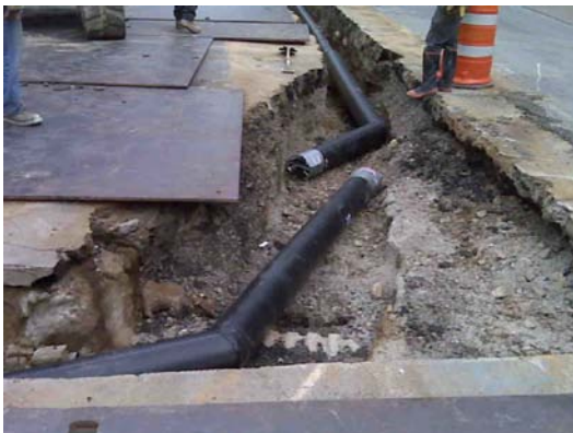
Ryman Auditorium Condensate Piping
