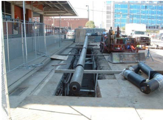
Manhole B to Symphony Condensate Line
