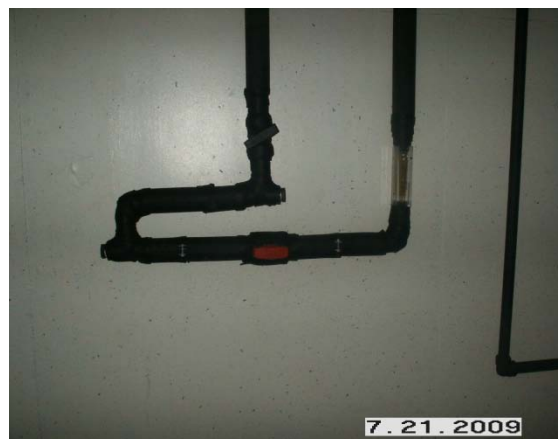
Chilled Water Coupon Station
