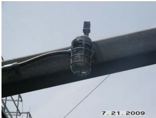
Cooling Tower Walkway Lighting
