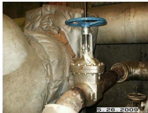
Manhole 23 New Steam Valve
