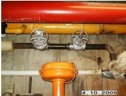
State Steam Tunnel PRV Bypass
