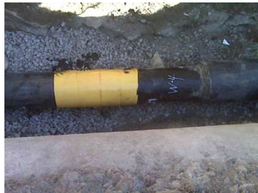
Ryman Auditorium Condensate Piping
