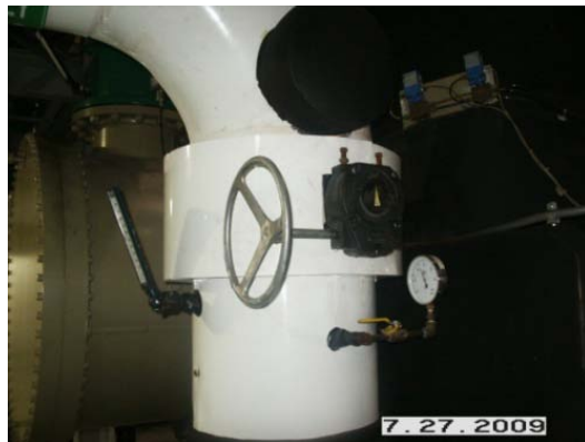
#3 Chiller Evaporator Outlet Valve
