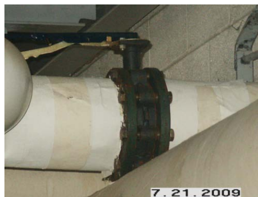
Cooling Tower Makeup Isolation Valve
