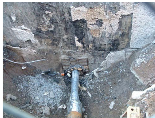
Citizen's Plaza Steam Piping Insulation
