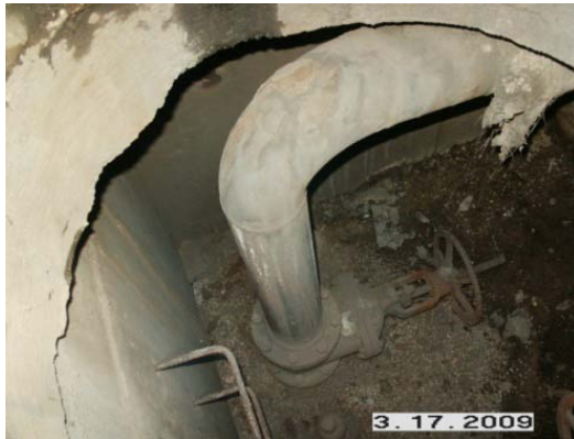
Manhole 6A Existing Steam Valve
