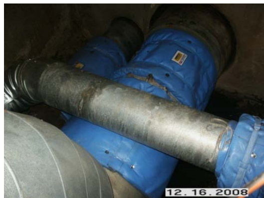
Manhole L Insulation
