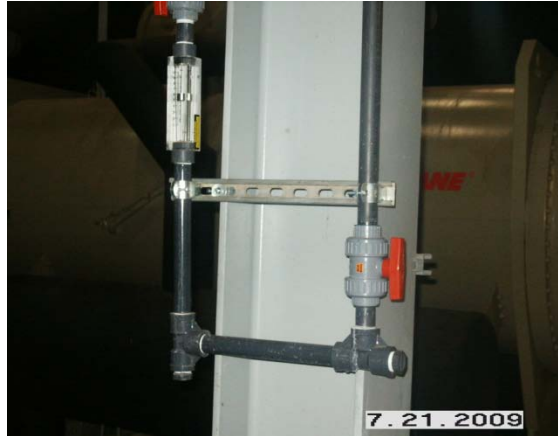
Condenser Water Coupon Station
