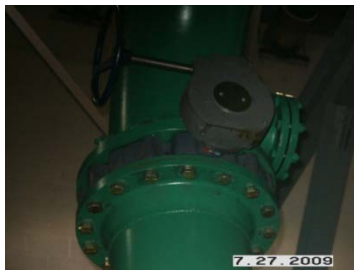
#5 Chiller Condenser Valve
