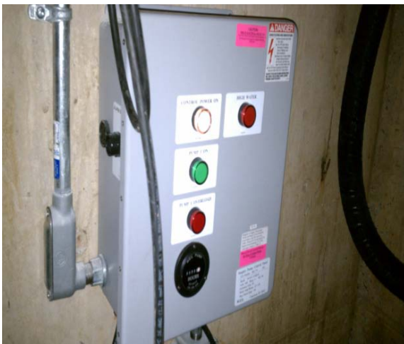
MH B Sump Pump Control Cabinet
