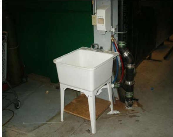
Maintenance Shop Sink
