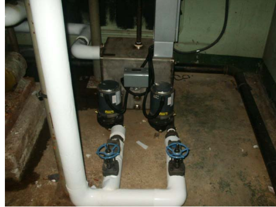
Municipal Auditorium Condensate Pumps
