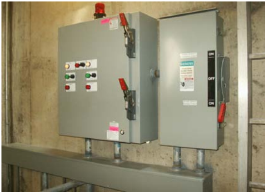
M/H 18 Sump Pump Control Panel
