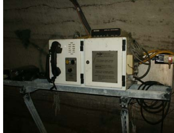
Tunnel Communication Base Station
