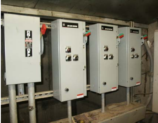
Tunnel Condensate Pump Disconnects
