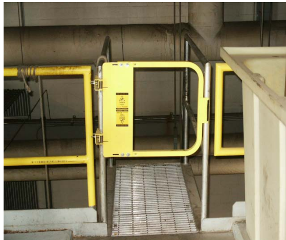
Mezzanine Level Safety Gate
