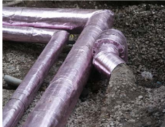
Steam, Condensate and ChW Piping to St. Mary's
