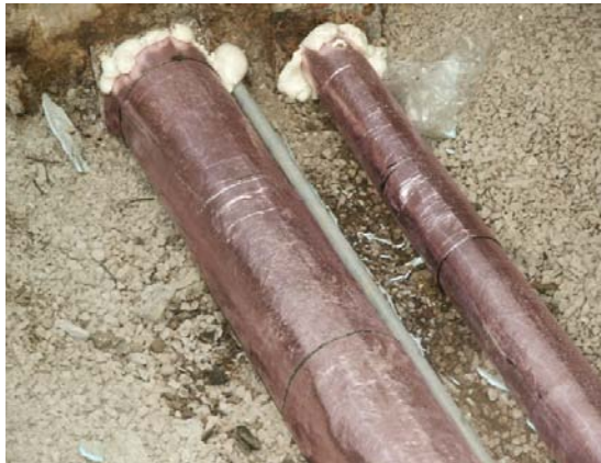
Steam & Condensate Piping to St. Mary's
