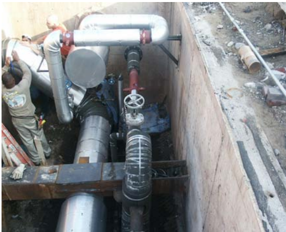
Manhole L Flood Damage Repairs
