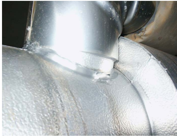
Manhole B2 Insulation
