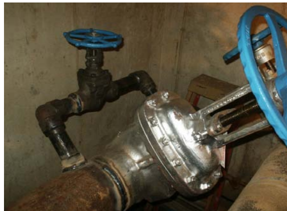
Manhole B4 Steam Isolation Valve for MCCC
