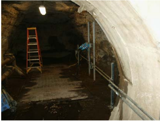
M/H 18 Sump Pump Electrical Connections
