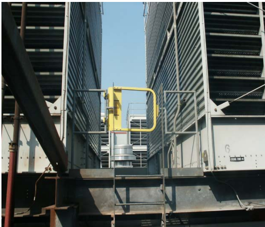
Cooling Tower Safety Gate
