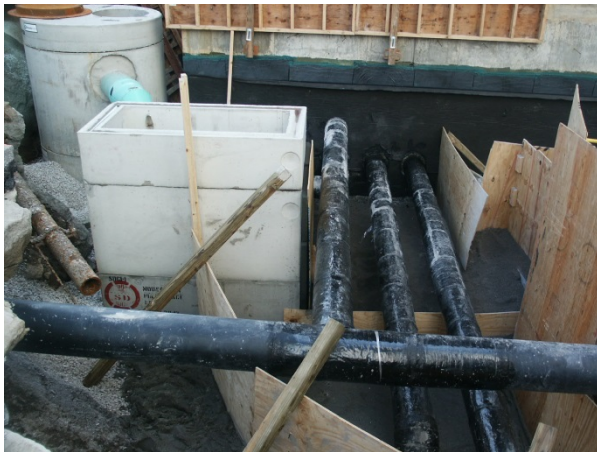
Service lines entering building on Molloy Street
