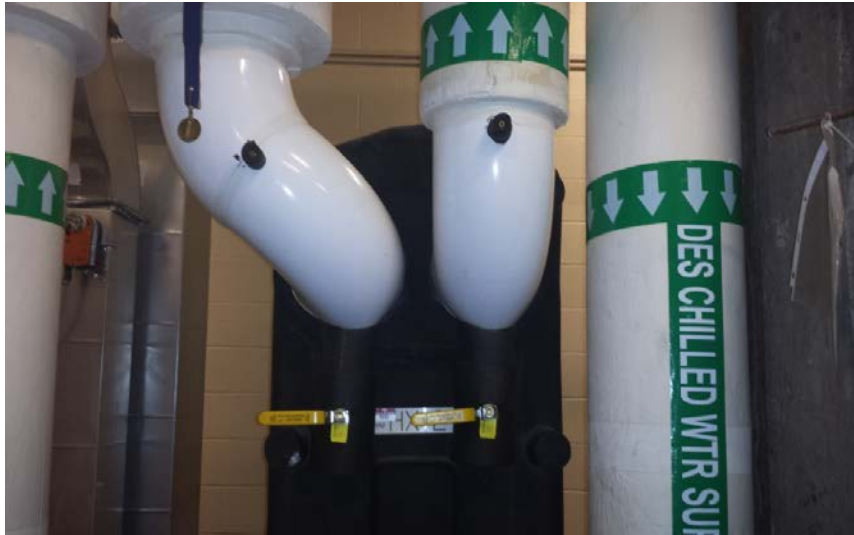
Courthouse HX Drain and Backwash Valves
