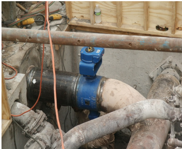
Manhole 10 Steam Isolation Valve
