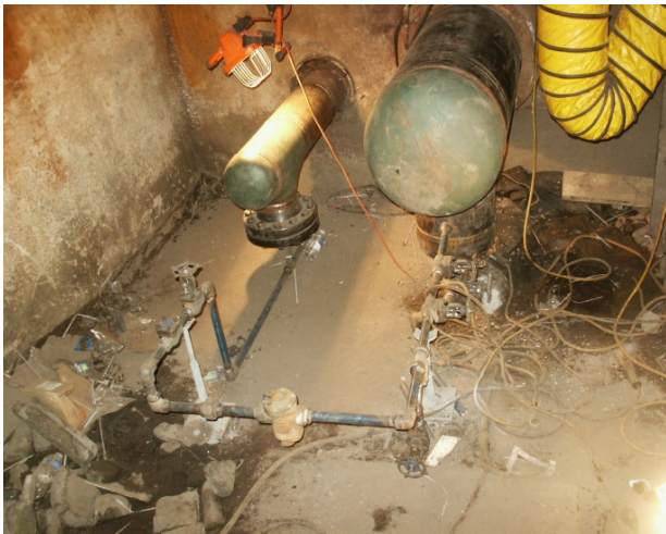
Manhole 2 Trap Assembly Capped Steam and Condensate lines
