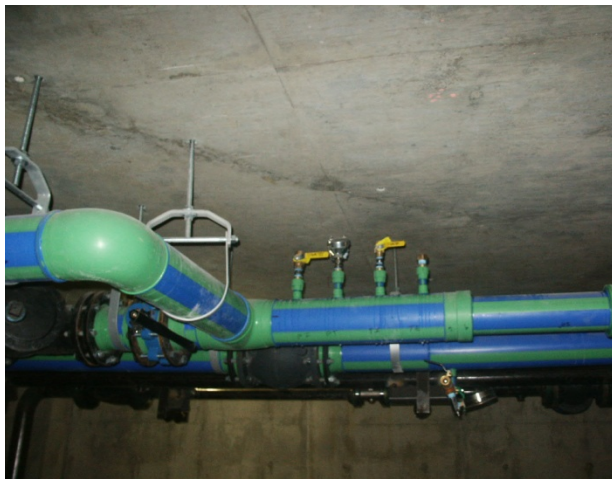
Hyatt Place Metering Devices
