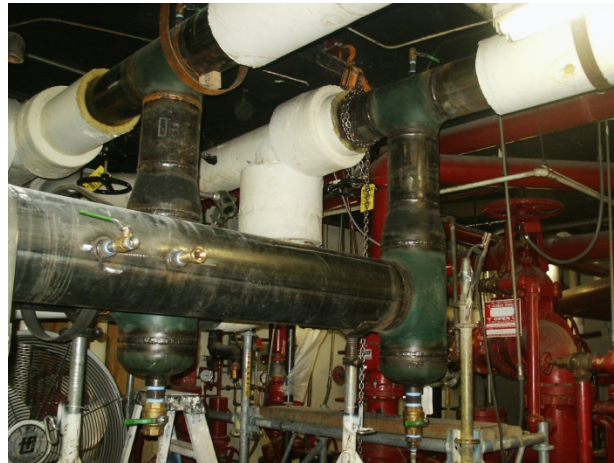
Sheraton Hotel Interior Chilled Water Piping
