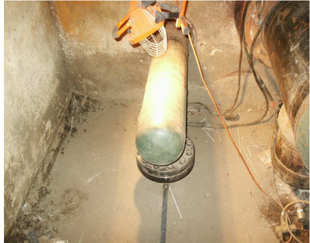
Manhole 2 Condensate Line with Sparge Tube Assembly
