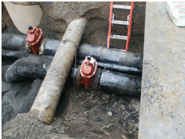
Sheraton Hotel Exterior Chilled Water Piping
