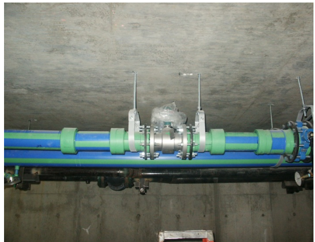
Hyatt Place Metering Devices
