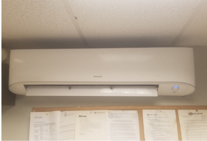
Control Room HVAC unit
