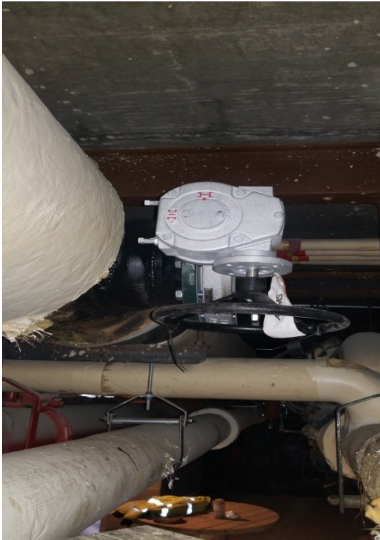
5 th & Broadway Chilled Water Supply Connection
