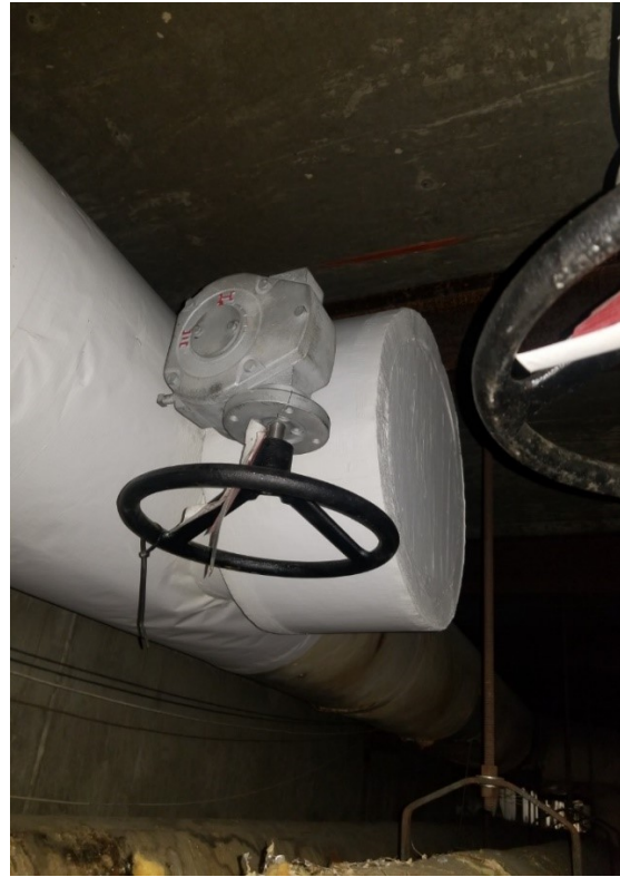
5 th & Broadway Chilled Water Return Connection
