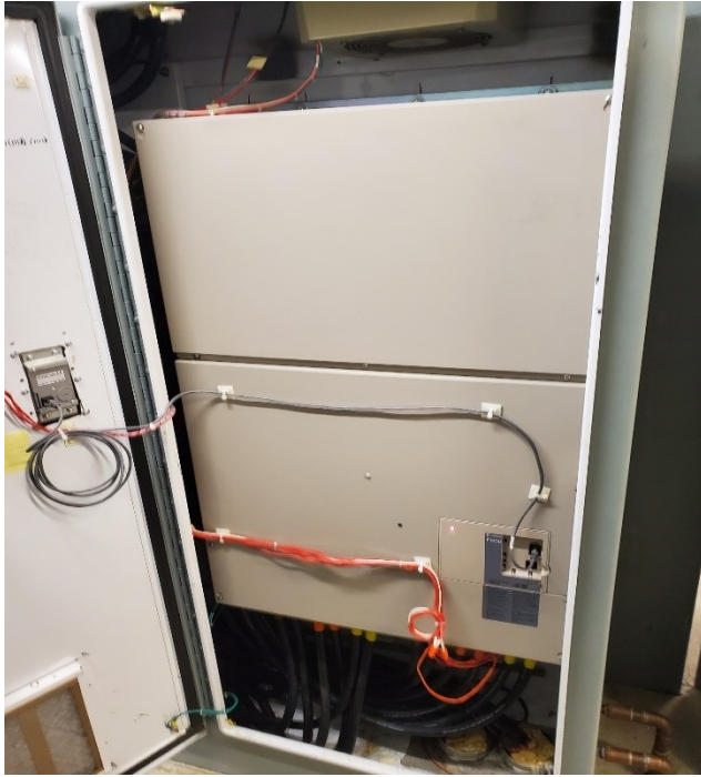
#6 Chilled Water Pump Variable Frequency Drive (VFD)
