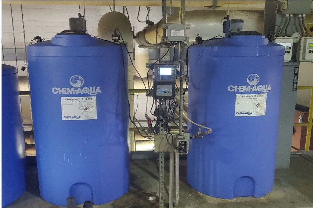
New Chemical Tanks and pumps
