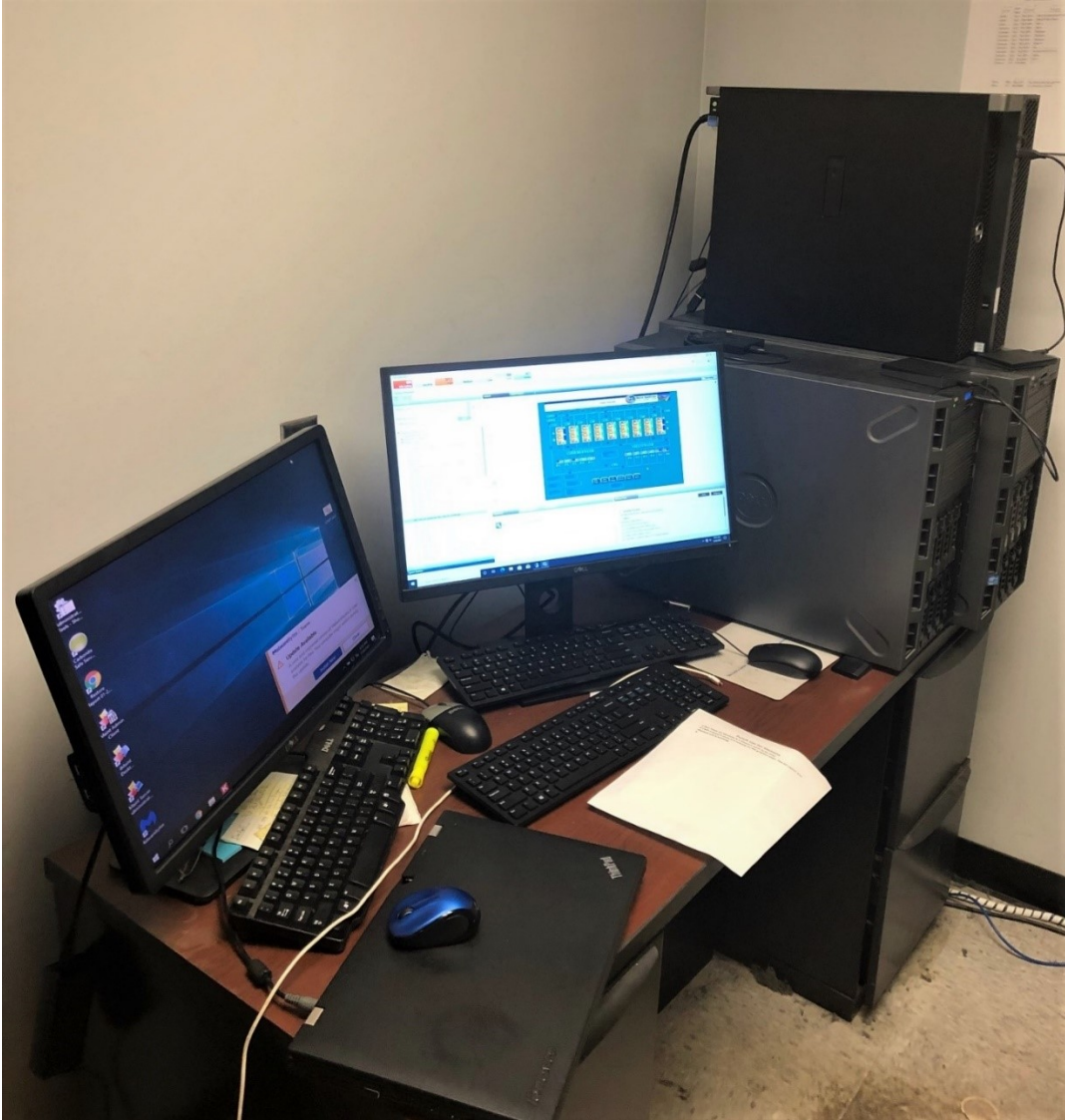
Siemens Control System Upgraded from Apogee Insight to Desigo CC (New Server)
