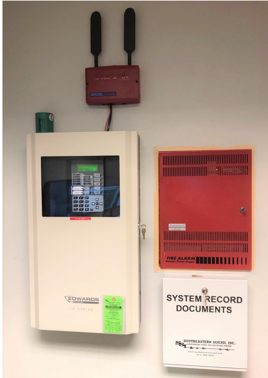
Fire Alarm System Upgraded (new panel)
