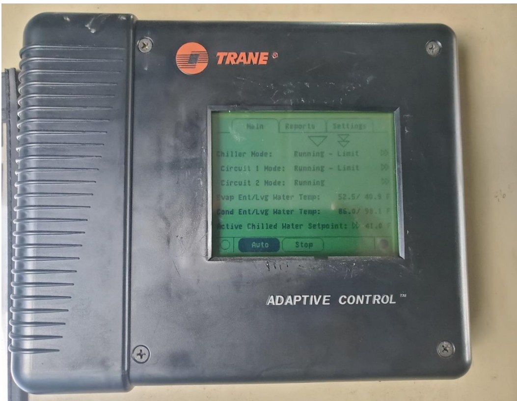
# 9 Chiller Panel Controller
