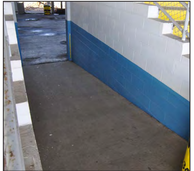
Steep access ramps to access ADA viewing deck
