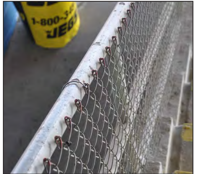
Exposed wire fence next to handrail
