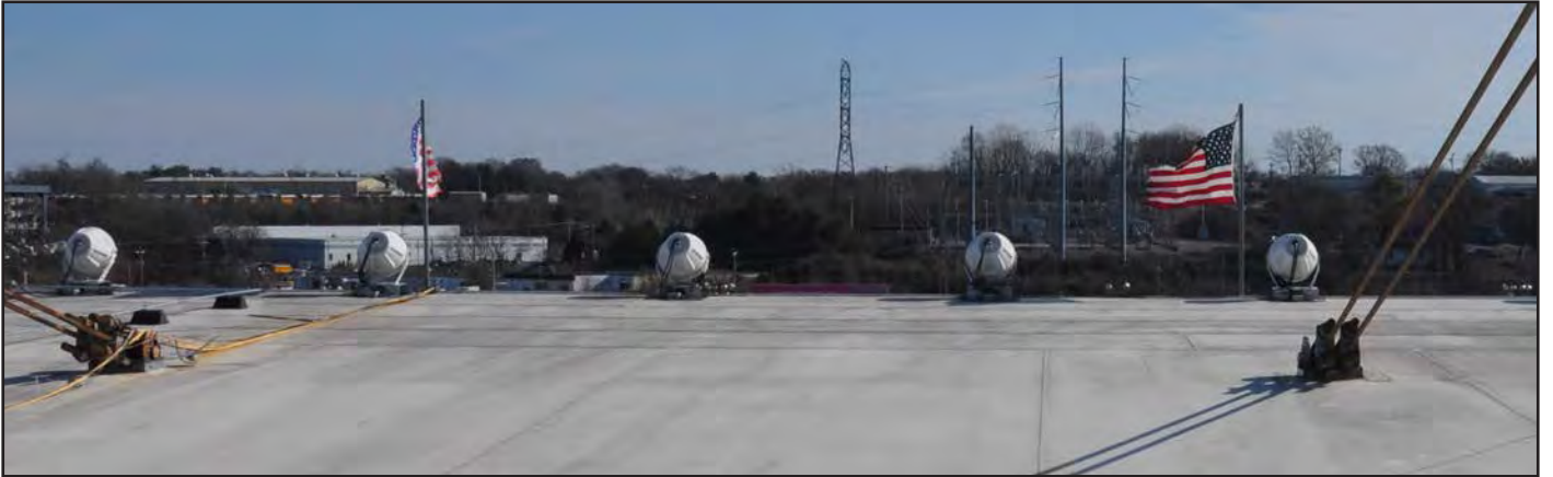
There is no visible mansafe or safety line system for working at height on the roof
