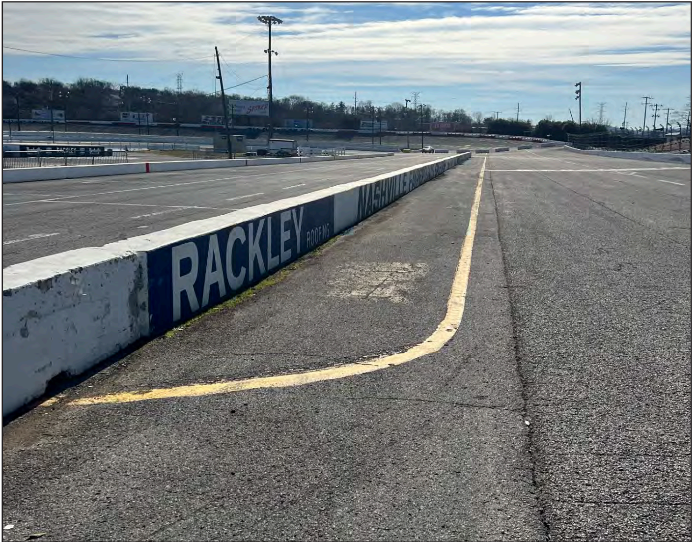
Moss and grass can be seen growing in front of the wall, indicating water ponding here after rainfall
