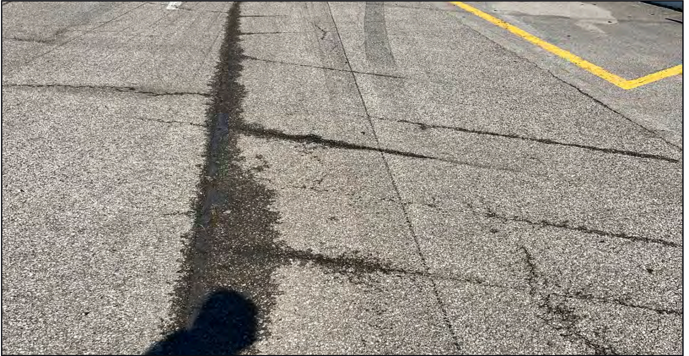
Existing drainage problems on track
