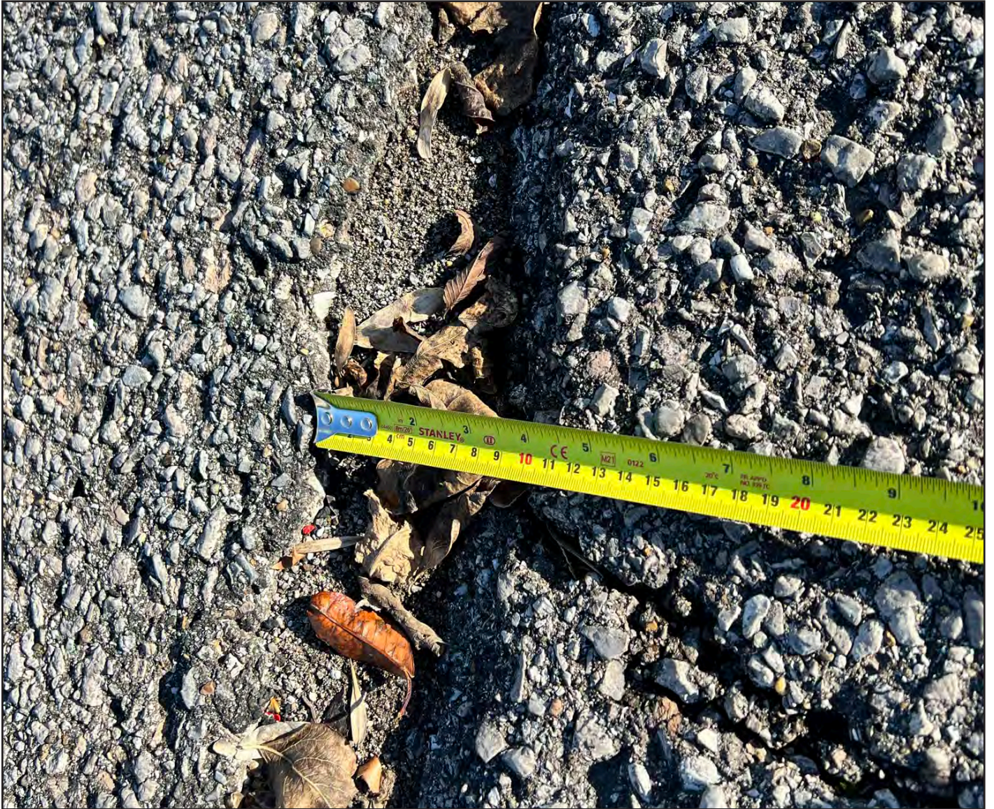
Cracking at joints which has subsequently spalled at the edges leading to a 4 inch gap in the asphalt.
