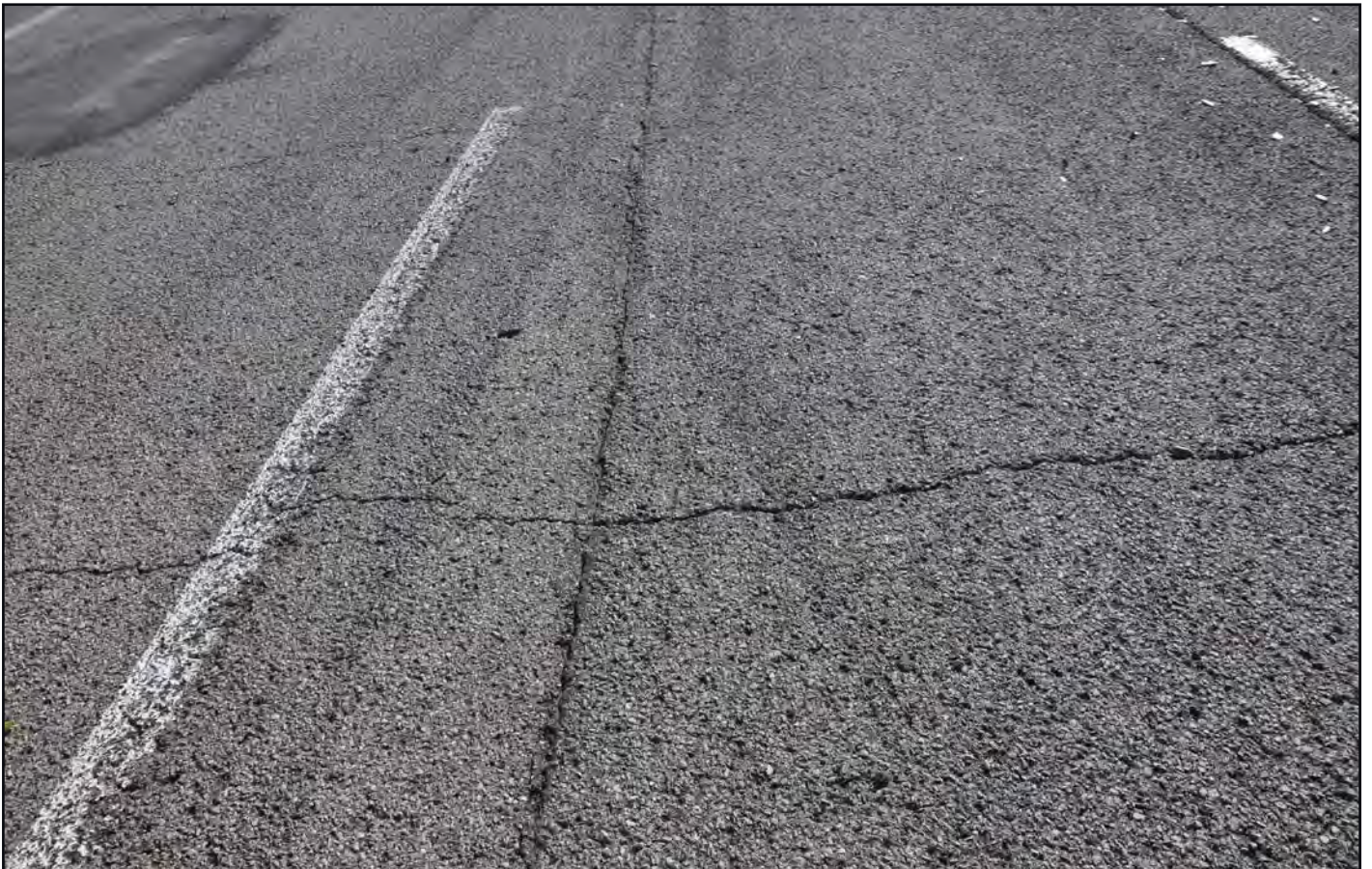
Visible cracking in asphalt
