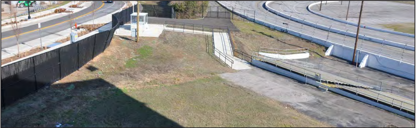
ADA Compliant ramp and viewing area, but does not connect to the rest of the venue
