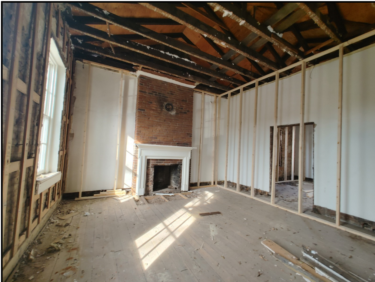
Example of interior shoring of a masonry building in preparation for foundation repairs.
