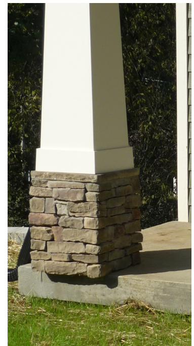
The depth of the stone veneer was not considered, leaving a porch pedestal hanging over the edge of the porch floor.
