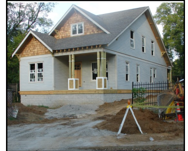
The rise in grade on this lot was not considered, resulting in a foundation significantly higher in the front than what the MHZ approved. Contractors had to stop work in order to devise a solution.
