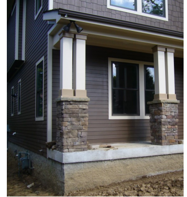
The foundation plans showed a porch depth of 4', the elevations showed a porch depth of 6' and the floor plans showed a depth of 8'. This homeowner now as a portion of their porch too narrow to be useful.
