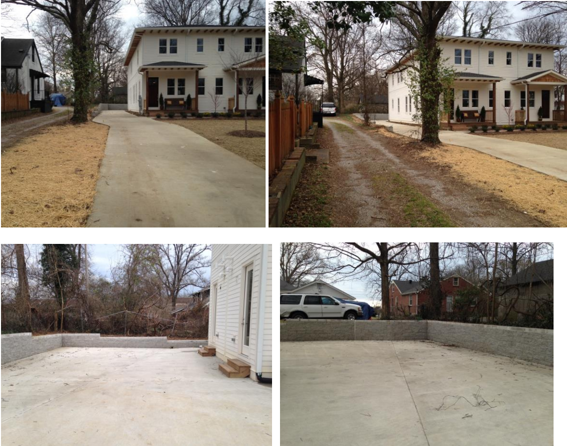
Figures 3 – 6 show the retaining wall and existing parking area at the rear of the lot.
