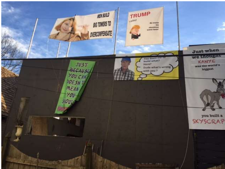
Rear of home with approved addition and with unapproved green-wall under construction. (MHZC does not review signage in this district.)
