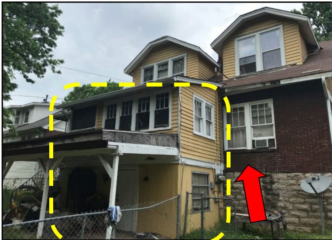
Figure 3: Rear elevation, box indicates addition to be removed, arrow indicates windows to be enclosed
