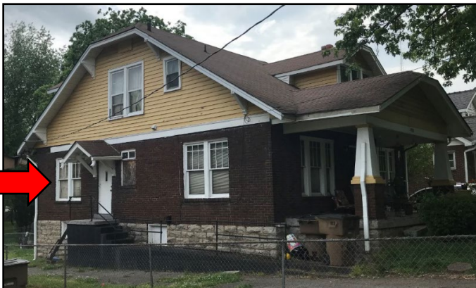
Figure 2: East elevation, arrow indicates windows to be shortened. Side door, hood and landing to be removed.
