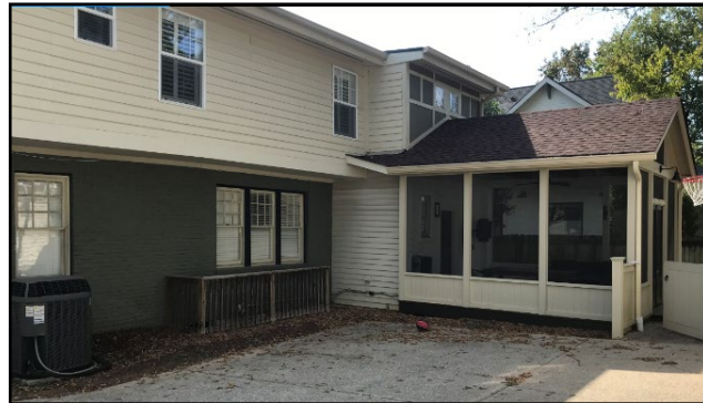
Figure 2: 1510 Paris Avenue – triple windows to be removed
