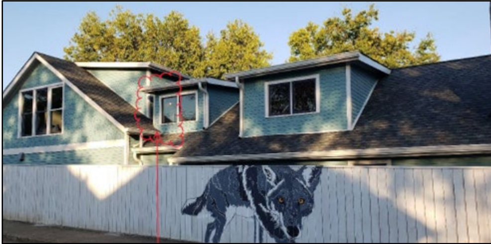
Figure 4: West elevation as constructed – red bubble indicates area of concern
