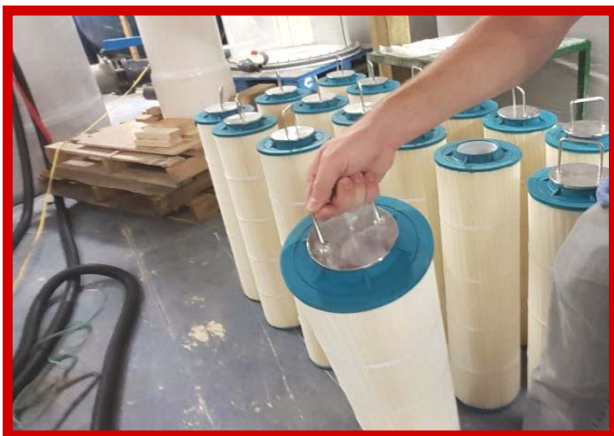
Once Cleaned Install Back Into the Vault. This Completes Maintenance. Ensure Access Lids are Properly Replaced.
