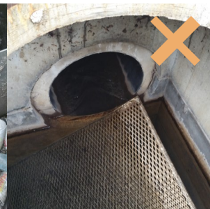
Trash screen displaced
