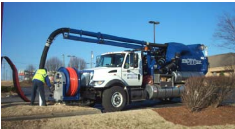
Metro has to clean grease from sewer lines to prevent overflows.
