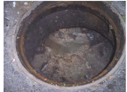
Sewer line blockage from grease.
