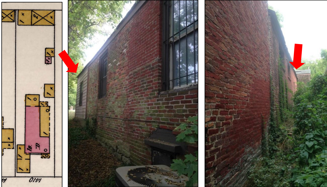
Figure 4 (left) is the 1897 map; Figure 5 (middle) is the addition to be demolished on the left side; and Figure 6 (right) is the addition to be demolished on the left side.
