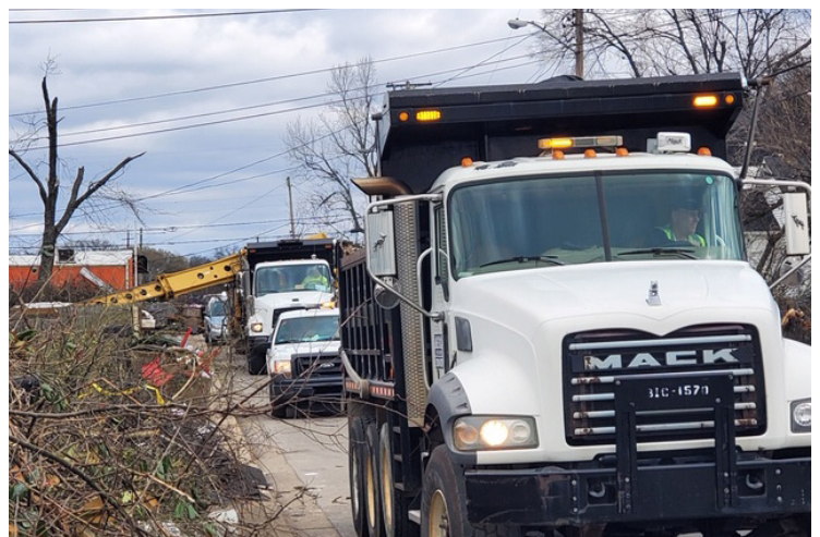
(Above) Trucks clearing debris after the tornado
