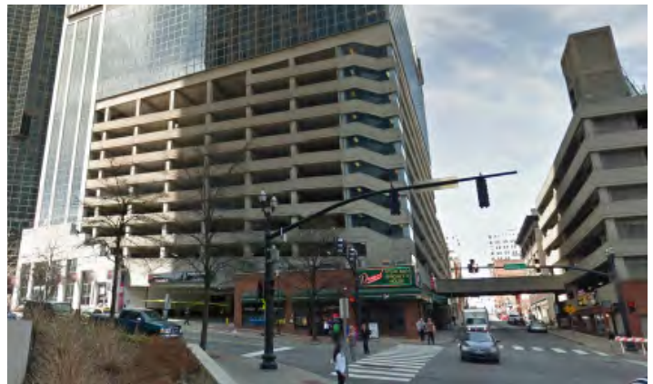
Inappropriate upper level facade treatment
