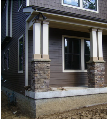
The foundation plans showed a porch depth of 4', the elevations showed a porch depth of 6' and the floor plans showed a depth of 8'. This homeowner now as a portion of their porch too narrow to be useful.
