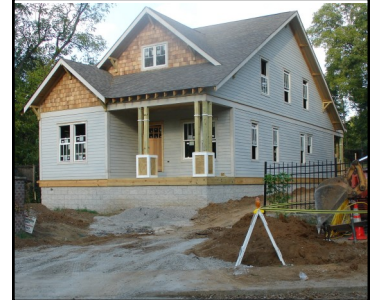
The rise in grade on this lot was not considered, resulting in a foundation significantly higher in the front than what the MHZ approved. Contractors had to stop work in order to devise a solution.
