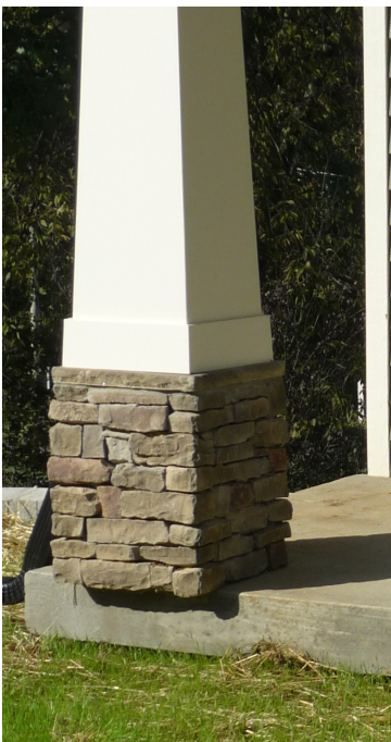
The depth of the stone veneer was not considered, leaving a porch pedestal hanging over the edge of the porch floor.
