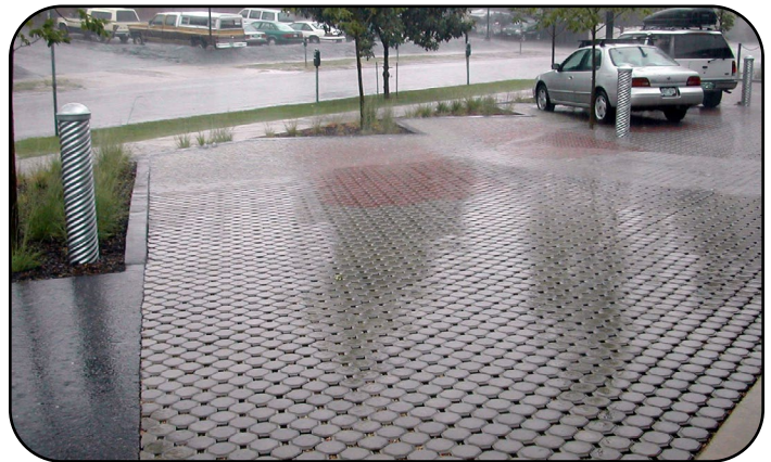
Permeable pavement in parking lot
