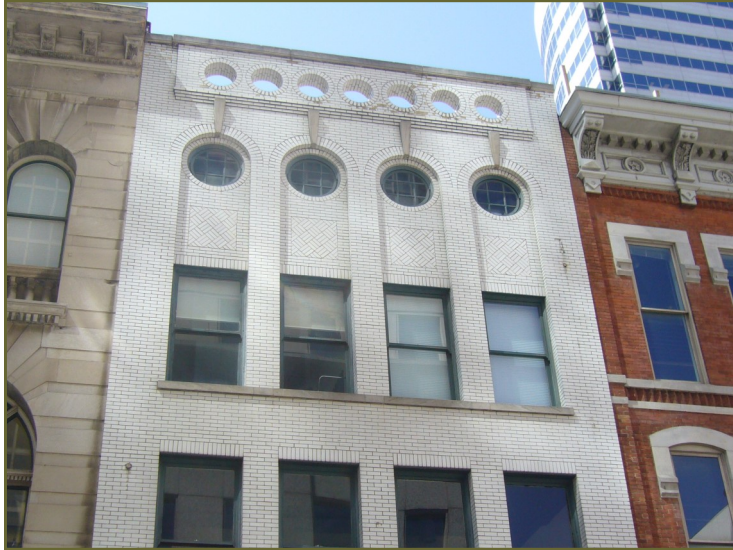
When the original window pattern is unknown, a simple one-over-one design for replacement single or double-hung windows is an appropriate choice.
