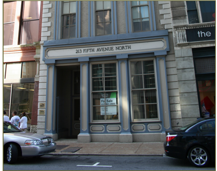
Historic storefronts such as this one at 213 Fifth Avenue North should be retained and, repaired, if needed, using materials that match the historic materials.
