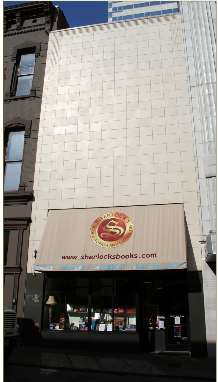
Property owners are encouraged to rebuild missing façade elements such as the windows and detailing removed at 235 Fifth Avenue.
