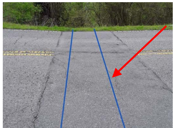
Patched Roadway Settlement/Failure
