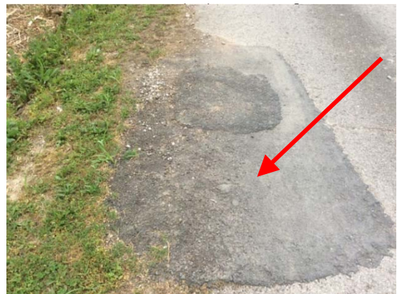
Patched Roadway Settlement/Failure
