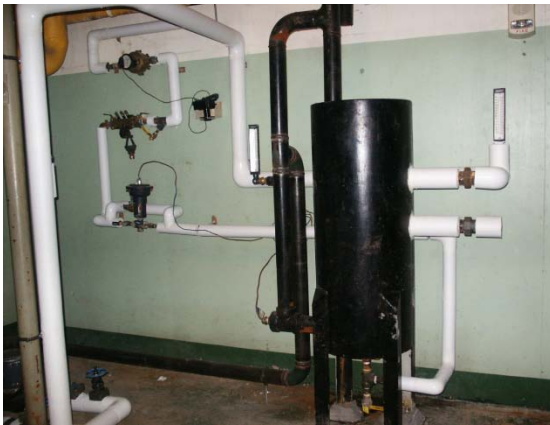
Municipal Auditorium Tempering Station
