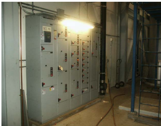
Lighting at MCC 4
