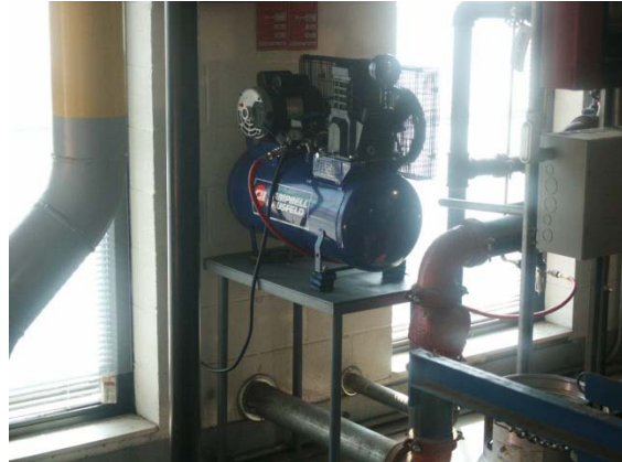
Plant Fire System Air Compressor
