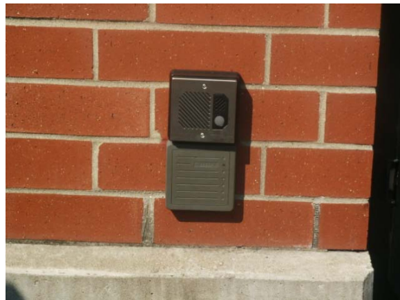
Plant Access Control Call Box
