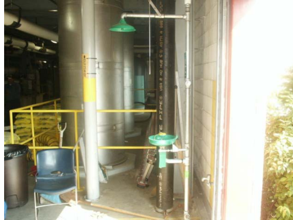
Eyewash and Shower Station
