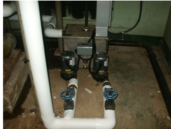
Municipal Auditorium Condensate Pumps
