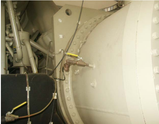
Differential Pressure Switch Isolation Valve (condenser)
