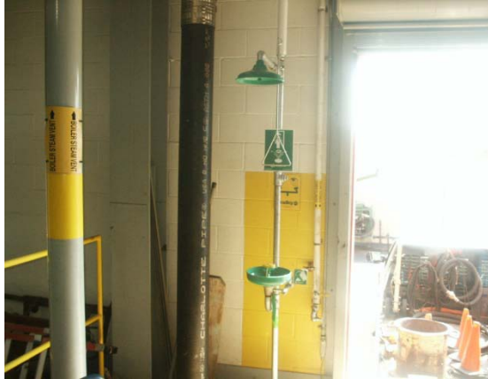
Eyewash and Shower Station
