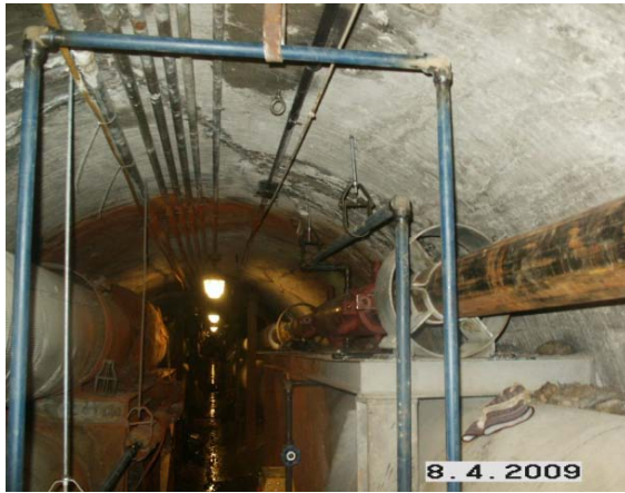
4 th Avenue Condensate Expansion Joint
