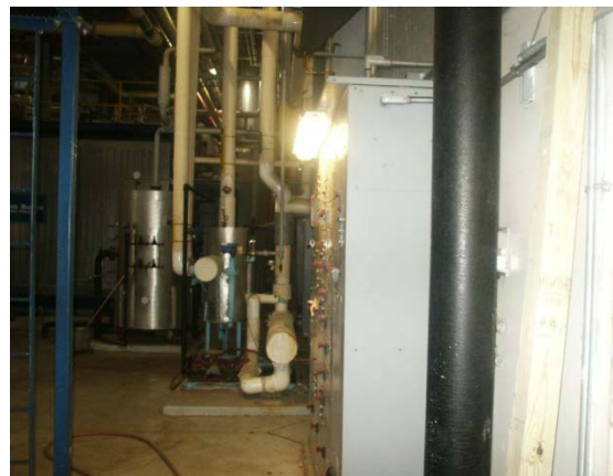
Lighting at MCC 4
