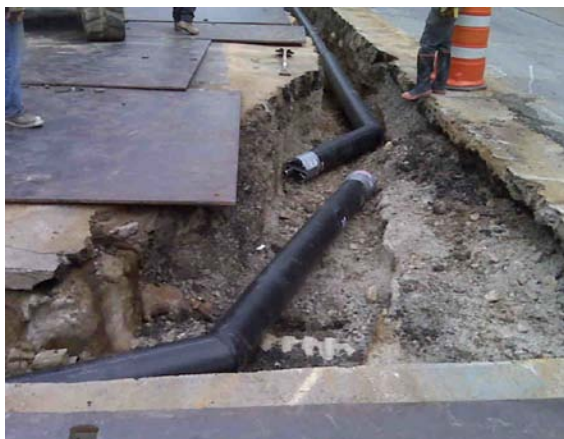
Ryman Auditorium Condensate Piping
