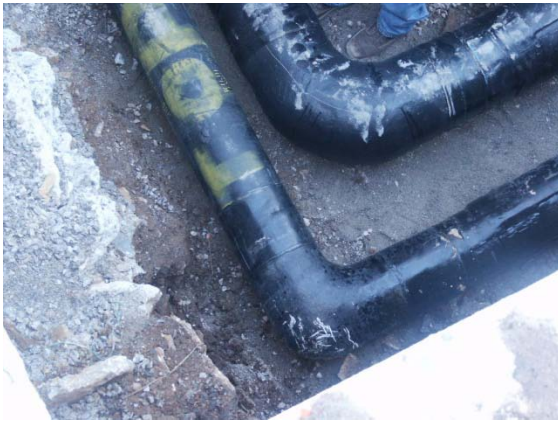
Wildhorse Steam & Condensate Service Lines
