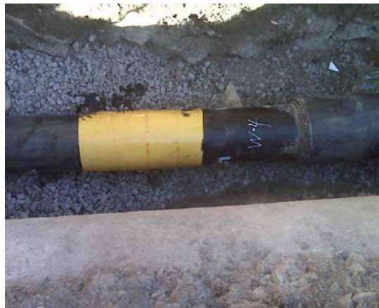
Ryman Auditorium Condensate Piping
