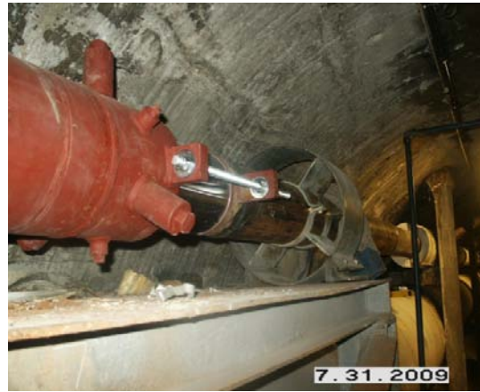
4 th Avenue Condensate Expansion Joint
