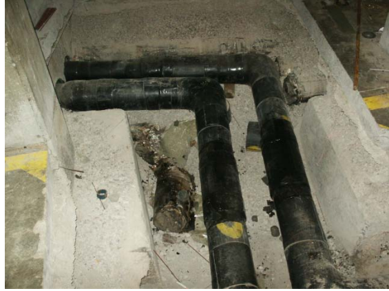
Wildhorse Steam & Condensate Service Lines
