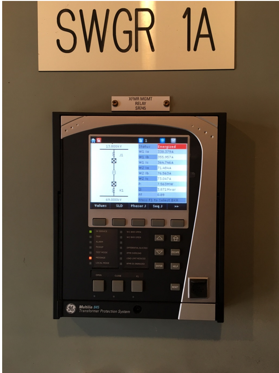
Upgraded Relay on Transformer 1A from 745 to 845
