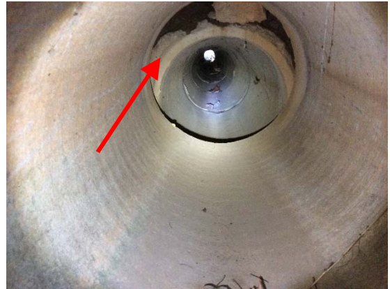
Pipe Separation & Settlement
