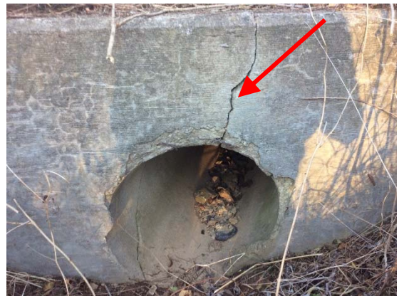
Concrete Damage @ Outlet Headwall
