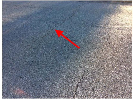
Pavement Settlement & Asphalt Cracking
