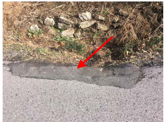
Section Loss & Corrosion
