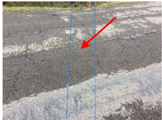
Seam Separation & Pipe Collapse
