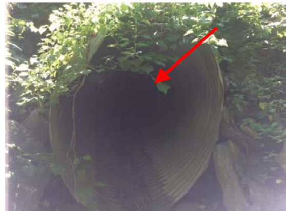
Deformed Pipe @ Outlet
