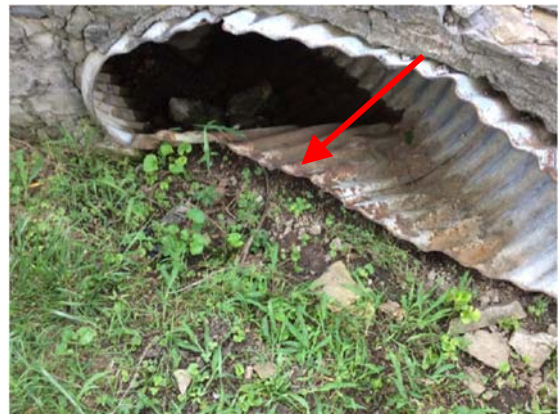
Deformed Pipe @ Outlet
