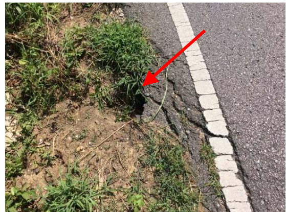
Partial Pipe Collapse w/ Heavy Corrosion
