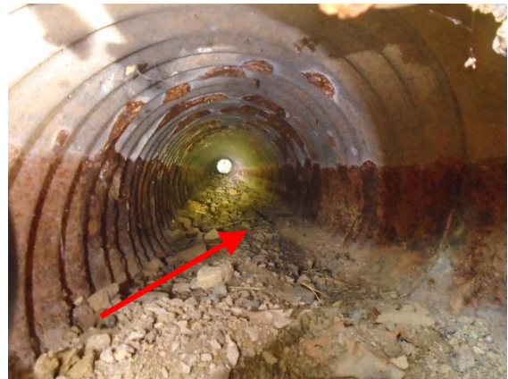
Heavy Corrosion w/ Areas of Section Loss
