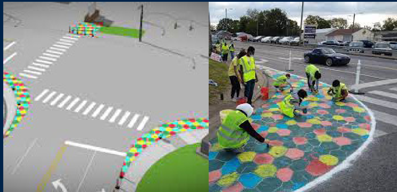
In 2021, the Civic Design Center, in partnership with the Nashville Youth Design Team and Walk Bike Nashville, implemented a temporary Glow in the Dark crosswalk at Dickerson Pike and Hart Lane. The project has since been upgraded with green, reflective paint to alert vehicles of pedestrians walking at night.
