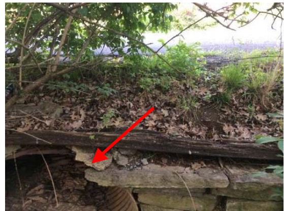
Failing Outlet Headwall
