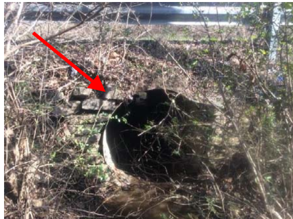
Headwall Failure w/ Steel Road Plate
