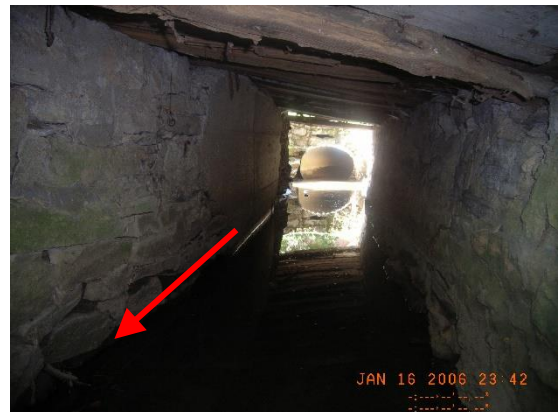
Scour w/ Associated Abutment Wall Destabilization
