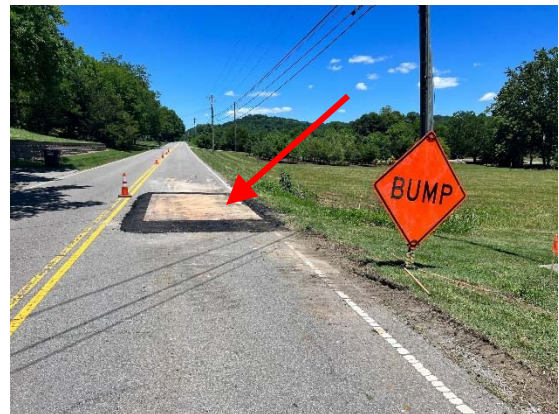
Roadway Failure w/ Steel Road Plate
