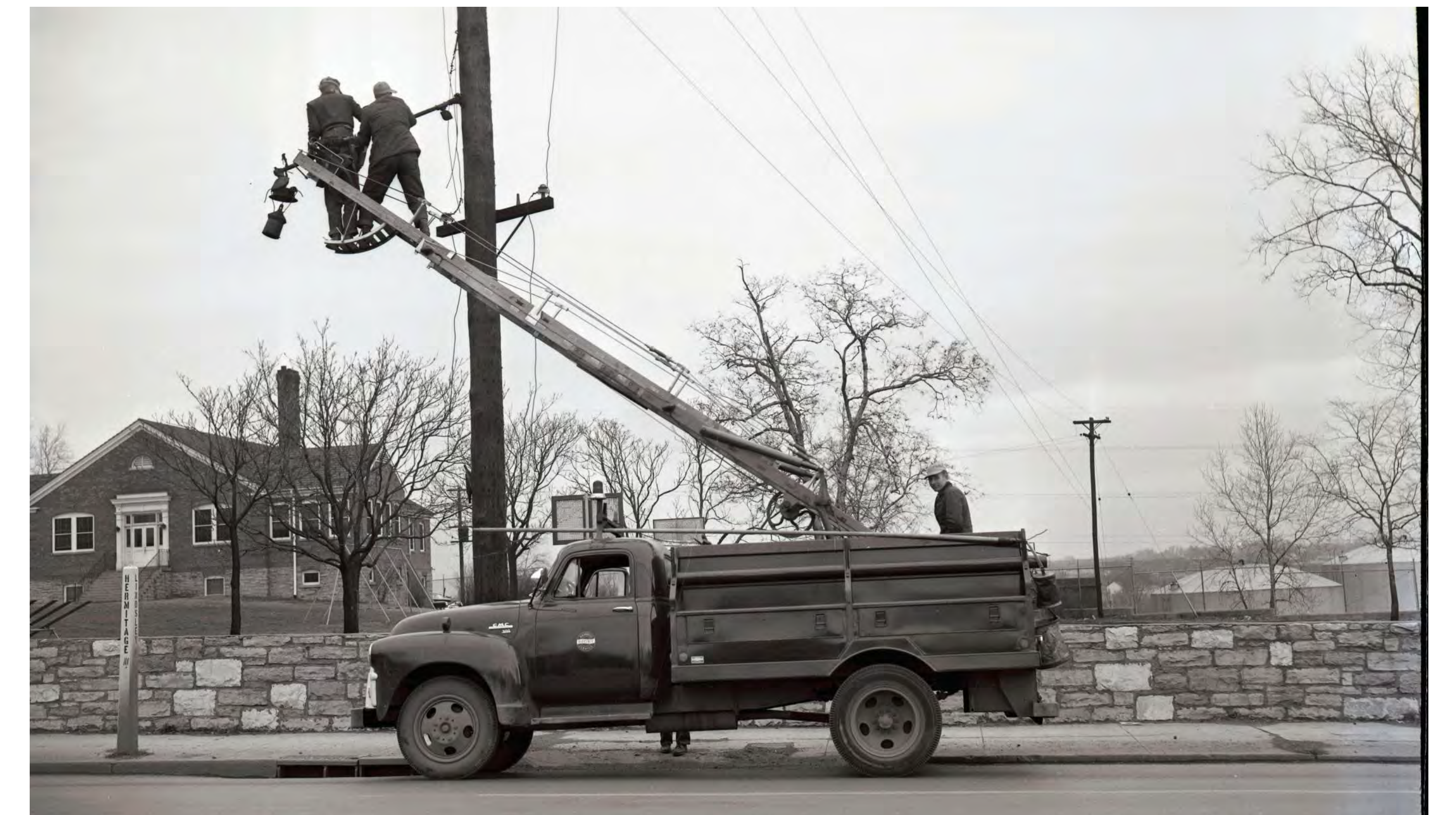
Nashville Electric Service doing repairs on Hermitage Avenue in the mid 1950's. The addition at 88 Hermitage is seen in teh background.
