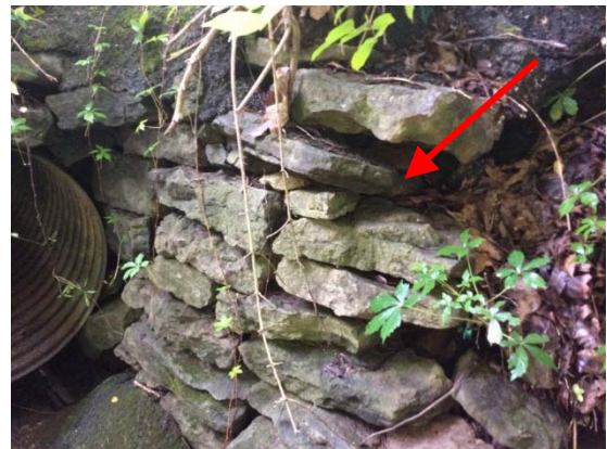
Failing Inlet Headwall
