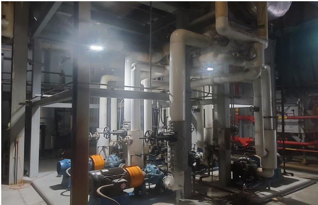
New Lighting at Boiler Feedwater Pumps
