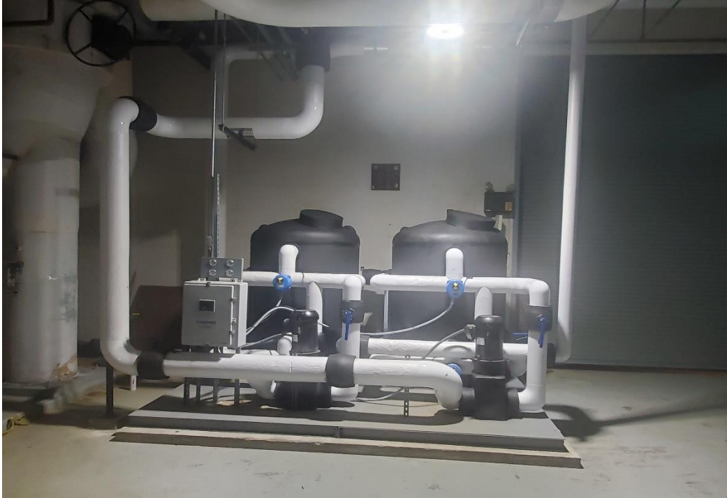
New Lighting at Side Stream Filter
